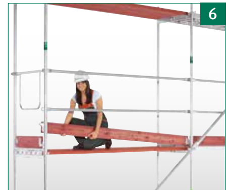
6 Assemble vertical frames and decks of the next level, then mount diagonal braces, guard rails and toe boards.
